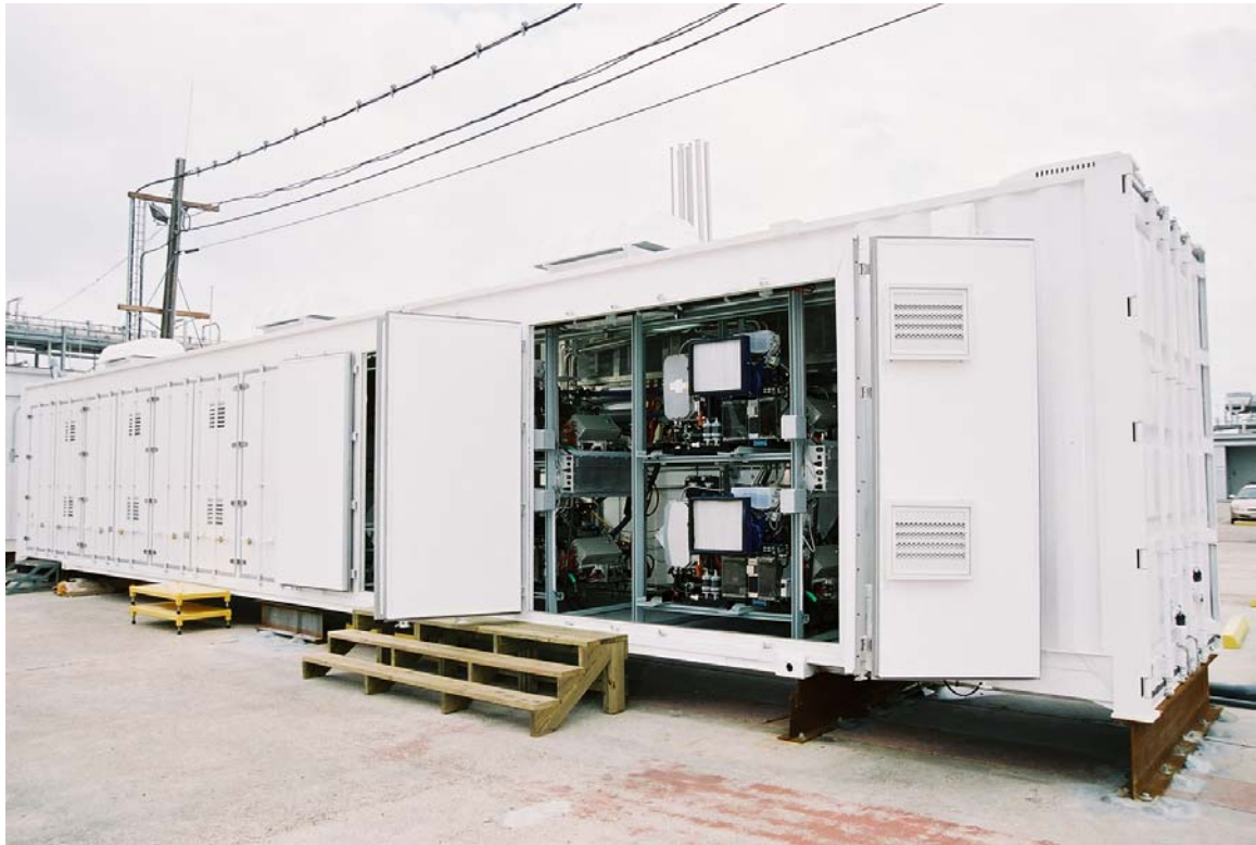
Picture of the trailer currently housing four new fuel cells installed as part of Phase 2 at the Dow Chemical plant in Freeport, Texas
